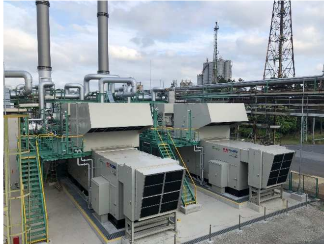
High Efficiency Gas Turbine Power Generators Reach Completion
