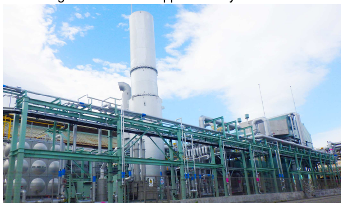
(The high-efficiency gas turbine power generator at the Omi Plant)
