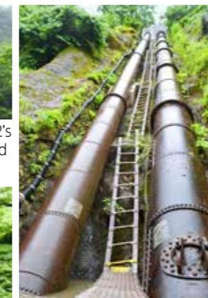
A closer look at the hydraulic steel pipes
