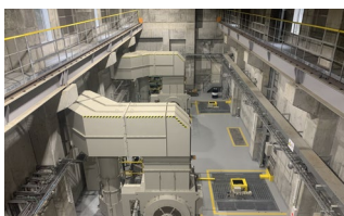
New Omi-gawa Hydroelectric Power Plant (interior)
