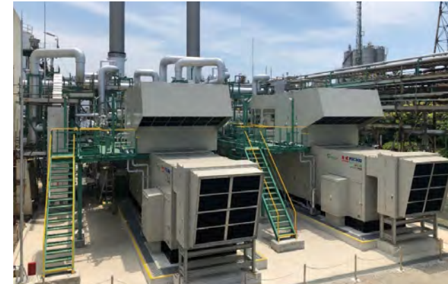
Gas turbine power generation facility at Chiba Plant, which started operation in June 2022
