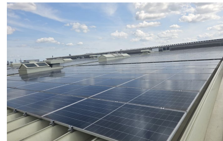
Solar power generation equipment that began operating at the Chiba Plant
