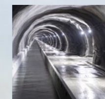
A water channel inside the Shin-Omigawa Power Plant. A road used for construction and maintenance runs alongside it.
