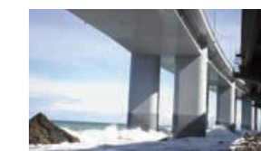
Desalination technology was applied to the Oyashirazu beach elevated bridge, which is part of the Hokuriku expressway
