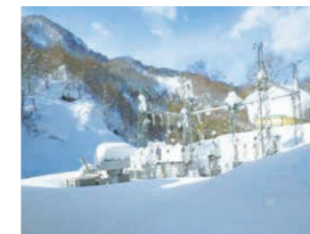
Power distribution facilities in winter
