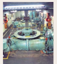
Inside the hydroelectric power plant
