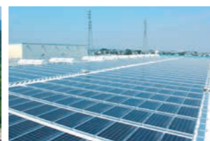
Mega solar power generation facility at the Isesaki Plant
