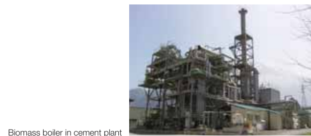
Biomass boiler in cement plant
