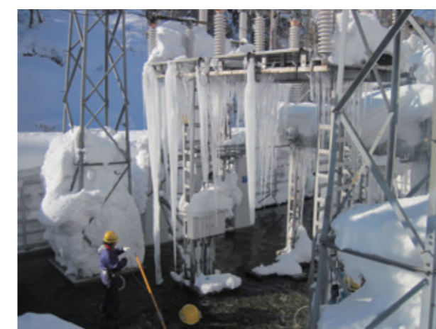
Large icicles on the Yokokawa Power Plant No. 1 switching station. Removing icicles, DENKA constantly works to maintain its facilities.
