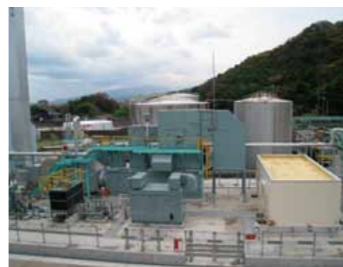
Tomi Gas Turbine at Omi Plant
