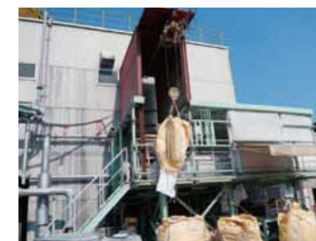
Soot and dust recycling facility at Omuta Plant
