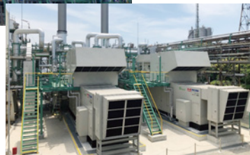
Gas turbine power generation facilities at the Chiba Plant, which began operation in 2022
