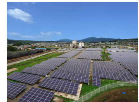
DENKA Solar Power Shibukawa
