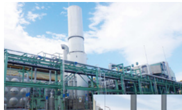
Gas turbine power generation facilities at the Omi Plant, which began operation in 2020
