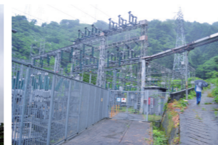
The Osawa Switching Station handles electricity from various power sources procured in-house and externally
