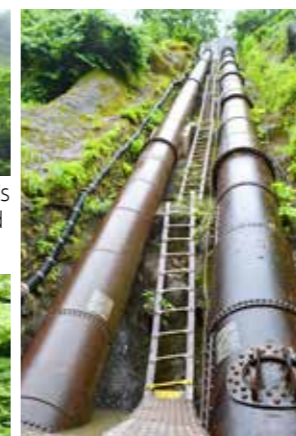
A closer look at the hydraulic steel pipes
