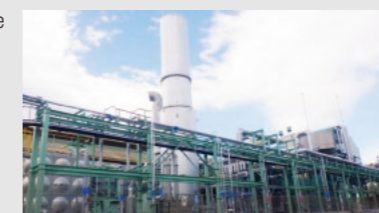
Construction of a high-efficiency gas turbine generator to reduce greenhouse gas emissions was completed at the Omi Plant in October.
