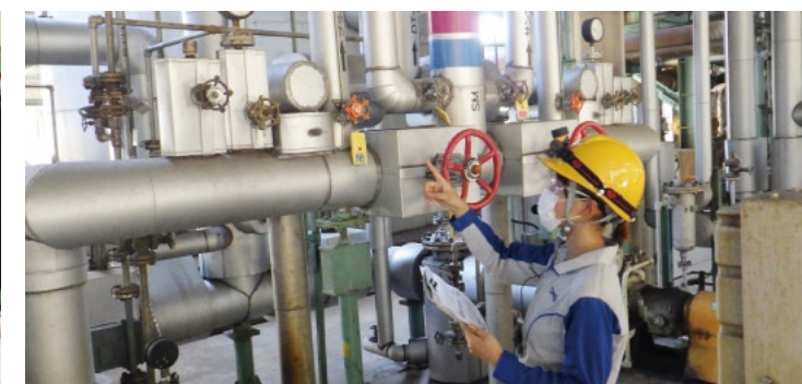
A worker checks pump discharge pressure in the plant. Providing workers with opportunities to gain experience in the field is important for human resources development.
