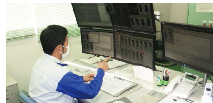
The DCS (Distributed Control System). Plant operations are constantly monitored and adjusted in the operations room.
