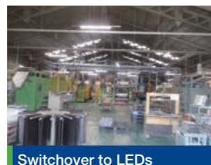
Switchover to LEDs
