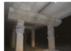
A pier of the Tohoku bullet train's elevated railway between Mizusawa-Esashi and Kitakami stations, which was damaged by the earthquake
