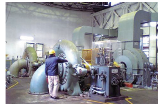
A generator at the Kotakigawa Power Plant with an output of 4,200kW
